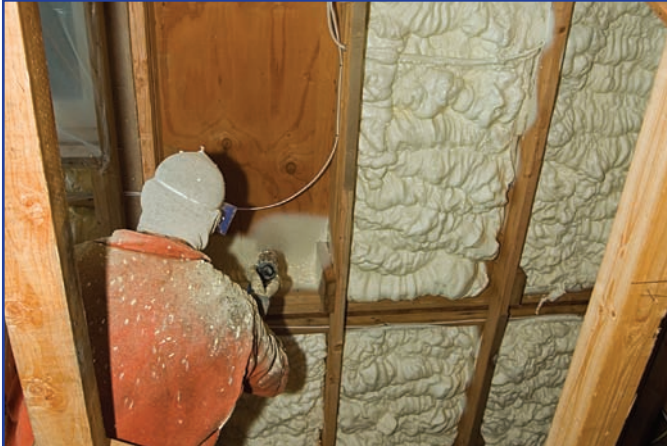
Icynene air-sealed all gaps and penetrations to minimize air leakage and help homeowners save up to 50% on energy costs.
