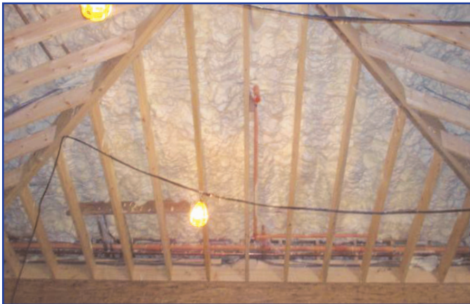
Icnene was sprayed into the cantilevered overhangs and roof assembly to prevent warm, moist air from coming into contact with cooler surfaces, minimizing the potential for condensation
