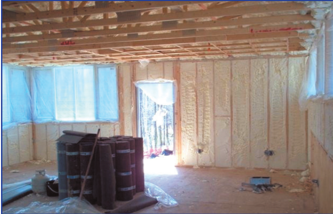
Icynene was so effective at minimizing air transport that it eliminated the need for additional sealing material.
