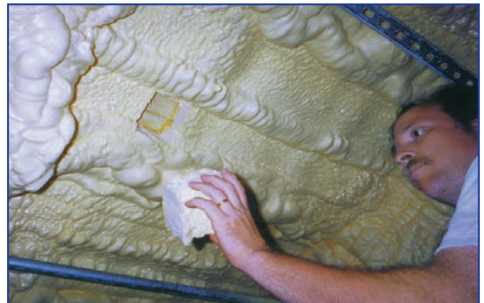
Wendell Porter demonstrates how the Icynene insulation is cool to the touch and prevents the metal roof deck from heating the interior air. On this June day, the exposed metal roof deck demonstration area was too hot to touch.
