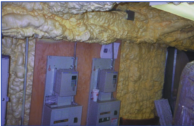
The Icynene foam was left exposed in the mechanical room, which is located in the upper area of the building.
