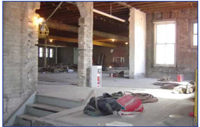
Once the interior was gutted, one of the first steps to creating a healthy, durable and energy-efficient building envelope was to have Icnene soft foam insulation and air barrier installed.
