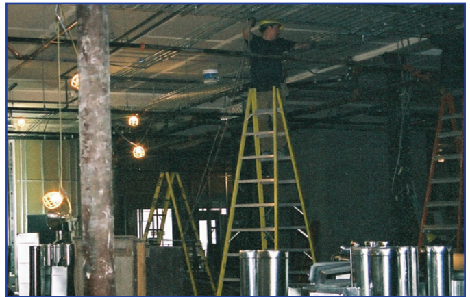
Icynene complements the new air quality system installed in the building, by locking out allergens and other pollutants and allowing building occupants to control the quality of the indoor air.
