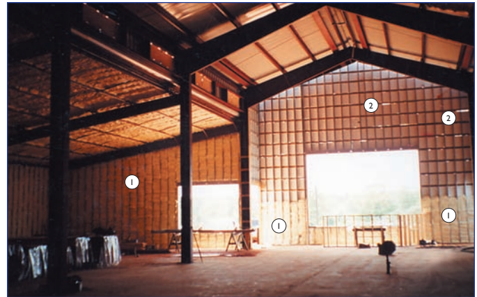
Icynene installed into the exterior wall cavities, prior to the installation of drywall. (1) Icynene sprayed area, (2) unsprayed area, note the gaps where air can freely pass through the wall. Daylight highlights these gaps.
